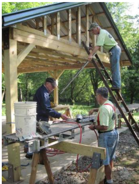
MYTC volunteers Bob Hoffman (left), Don Baker (right) and John Eisenbarth (on ladder) work to complete the Kenneth Frew Memorial Pavilion in the Queen Aliquippa Camp
